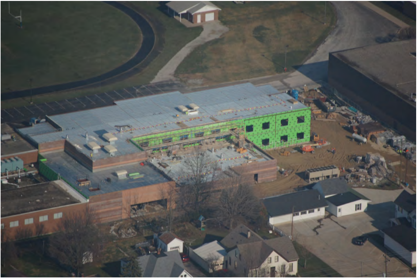
Aerial Photos of BIS construction site taken by Ray Call, submitted December 19, 2011
